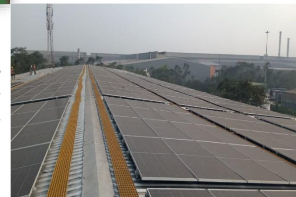
Rooftop Solar Capacity: 23 MW Installed Capacity: 13 MW
